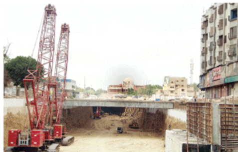
KARACHI: A view of construction work of Green Line Bus Service in Numaish area.—Online
